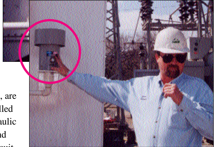
James Mitchell, NES supervisor--underground and substation, specifies Des-Case breather models CS-6 for NES oil tankers.
